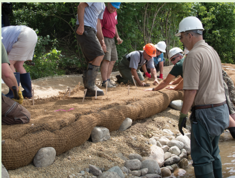
Figure 1. Workshop participants install a prefabricated soil lift at Kellogg Biological Station near Hickory Corners, Michigan, in July 2011. The participants were Certified Natural Shoreline Professionals (CNSPs) who earned continuing education units by installing traditional and prefabricated ESLs for this comparison study during a one-day workshop. You can watch a brief video about the installation at www.shoreline.msu.edu/shorelinemgt/natural-shoreline-constructing-encapsulated-soil-lifts/ .
