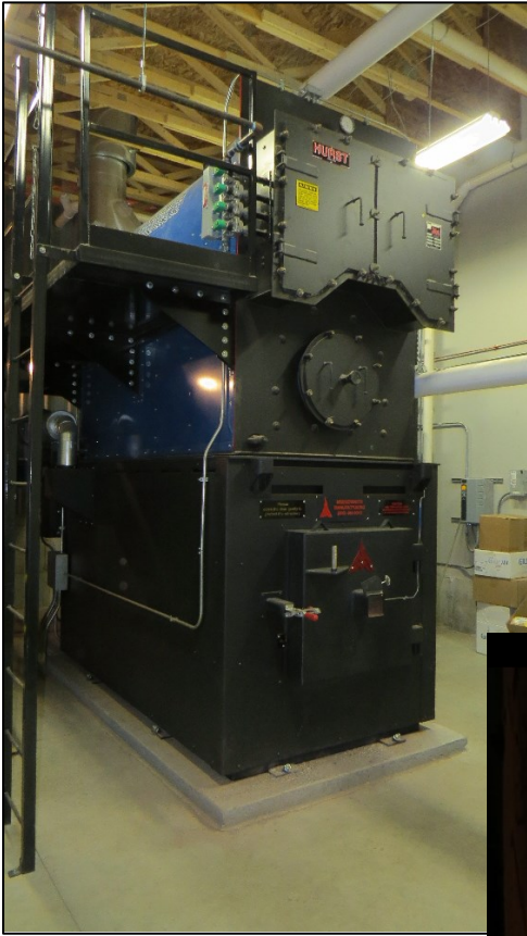
Combustion chamber and overhead boiler.
