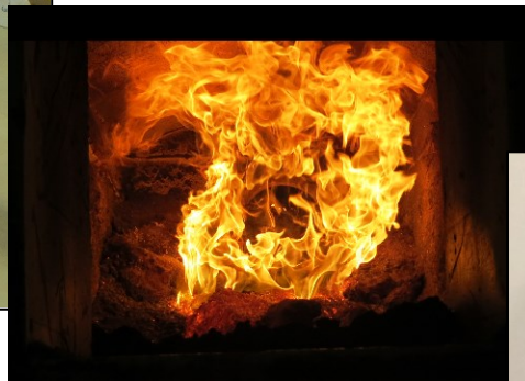
Fire in combustion chamber.
