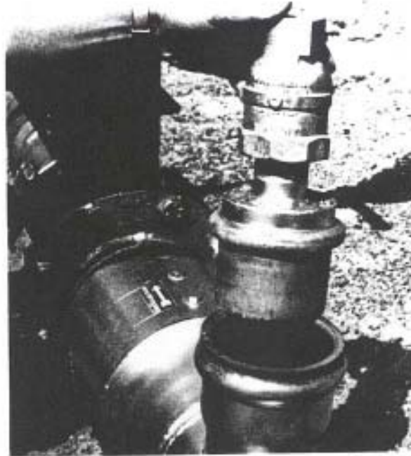
Removable vacuum relief valve serves as a port to inspection check valve.
