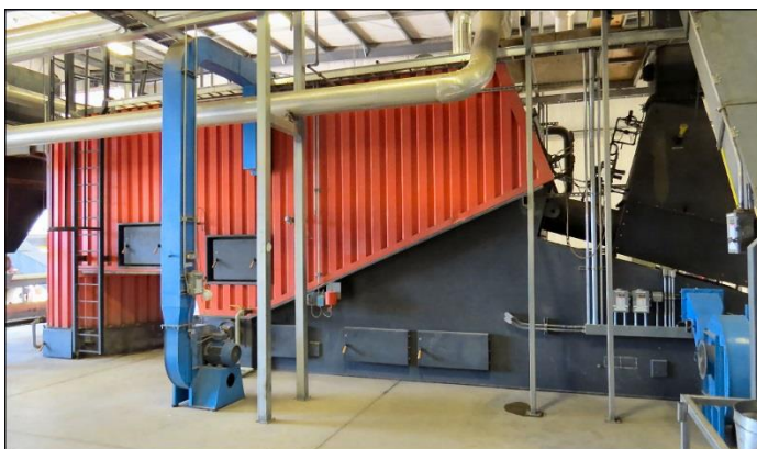
Vyncke boiler, 10 million btu and 3 megawatt capacity.
